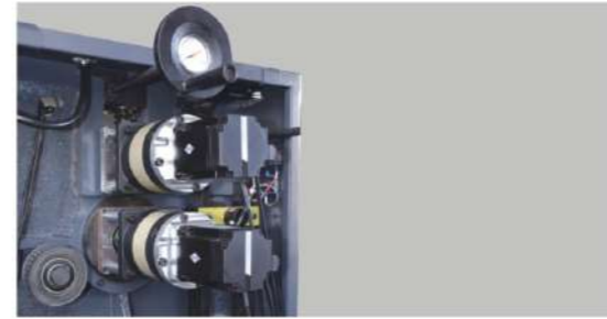
涂布电器传动 Coating electrical transmission
